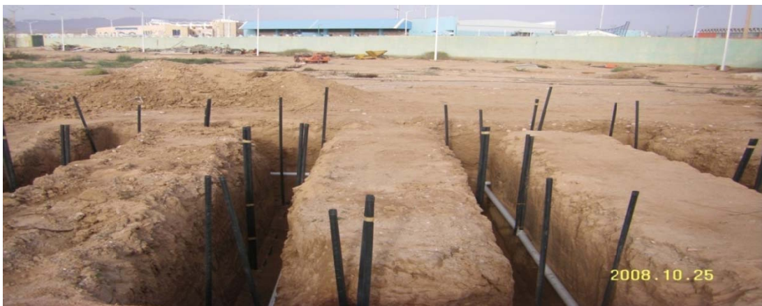
Fig.(I-12) : Experimental site consisting of trenches for installation of the geothermal air/sol exchanger. [5].
